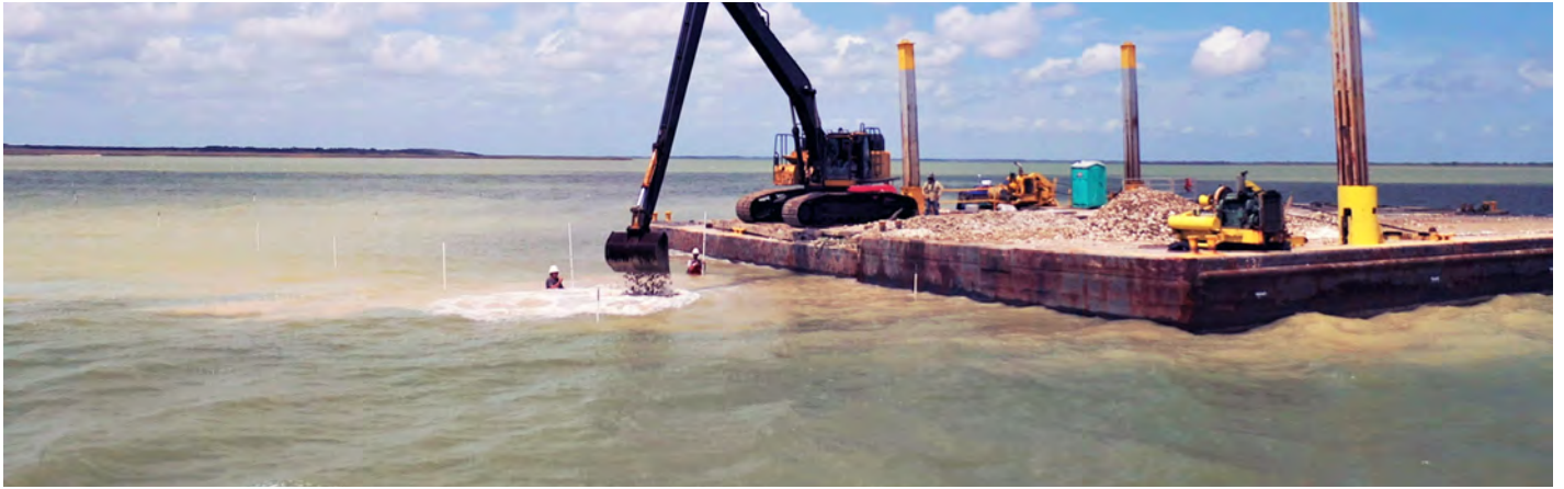
Materials staged and ready for Phase III of the St. Charles Bay Big Tree Unit Living Shoreline Oyster Restoration Project. Photo by John Blaha
