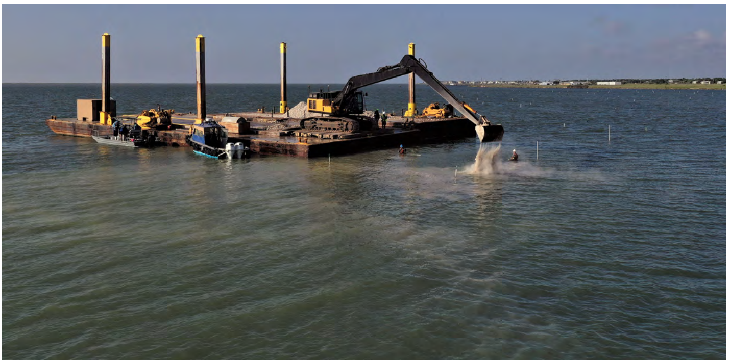
Contractors place rock cultch into the St. Charles Bay Big Tree Unit reefing area. Each reef bed is checked continuously through construction to ensure proper amounts of material are placed and settled properly.
