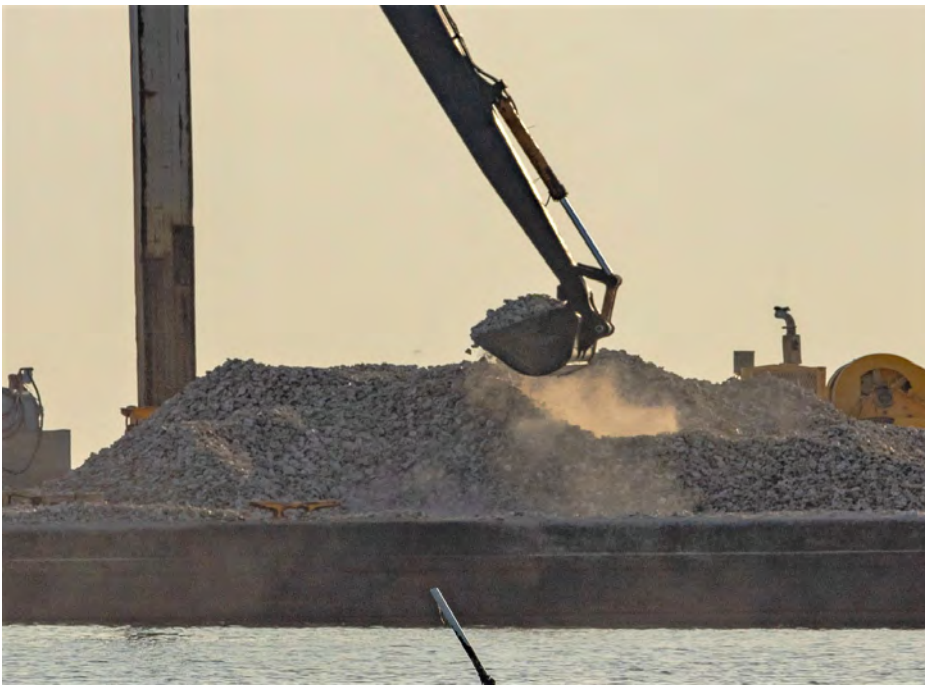
Derrick Construction puts the finishing touches on five reefs beds in St. Charles Bay Big Tree Unit reefing area. After the initial rock culch is layed, contractors then place a coating layer of recycled oyster shell from area restaurants and shucking houses. Photo Courtesy of Janae Evans
