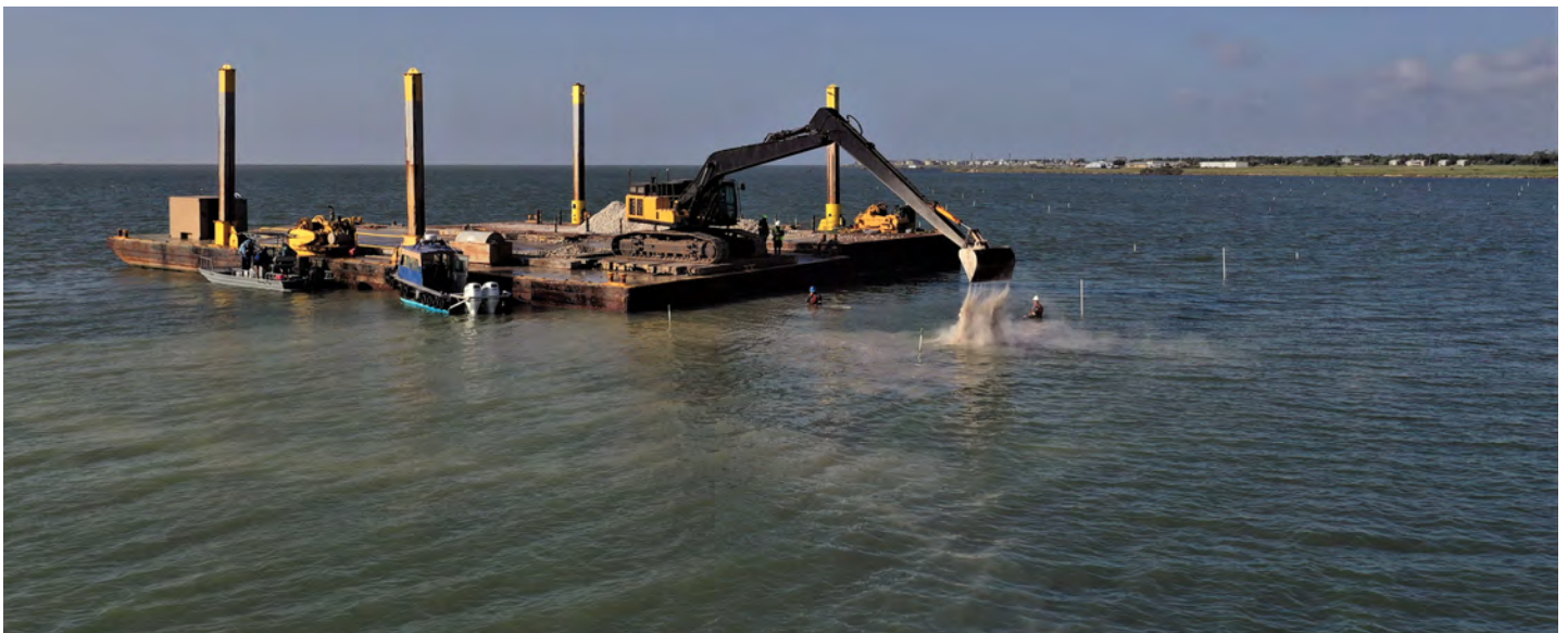
Contractors place rock cultch into the St. Charles Bay Big Tree Unit reefing area. Each reef bed is checked continuously through construction to ensure proper amounts of material are placed and settled properly.
